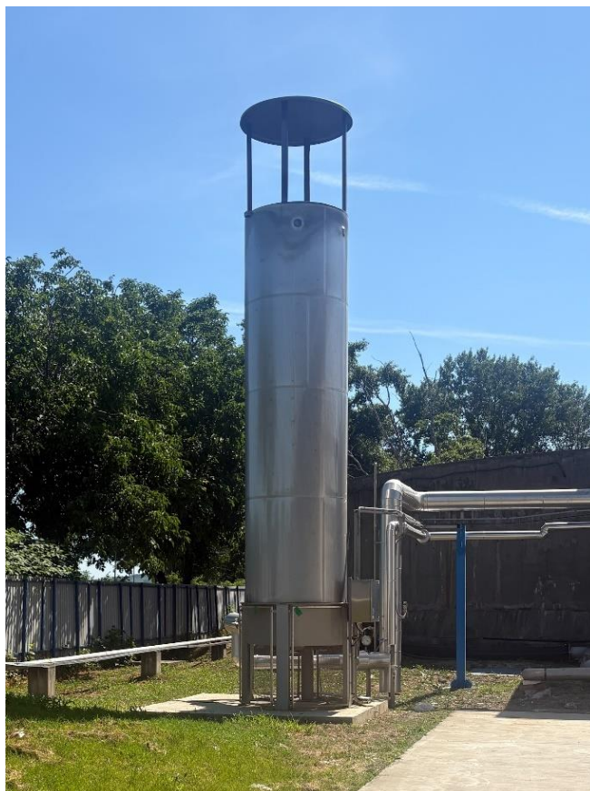
Figure 5. Newly installed flare in SWB
